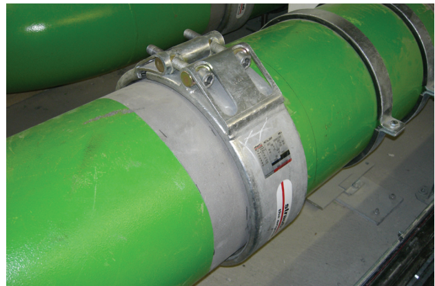
Cooling pipeline of an engine test facility with a working pressure of 6 bar and a temperature up to 60°C
